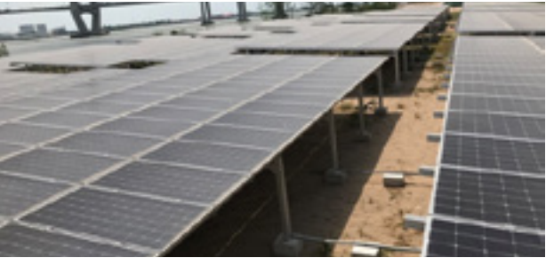
Image of a 500-KWP-capacity solar battery station in Con Au, Can Tho City
